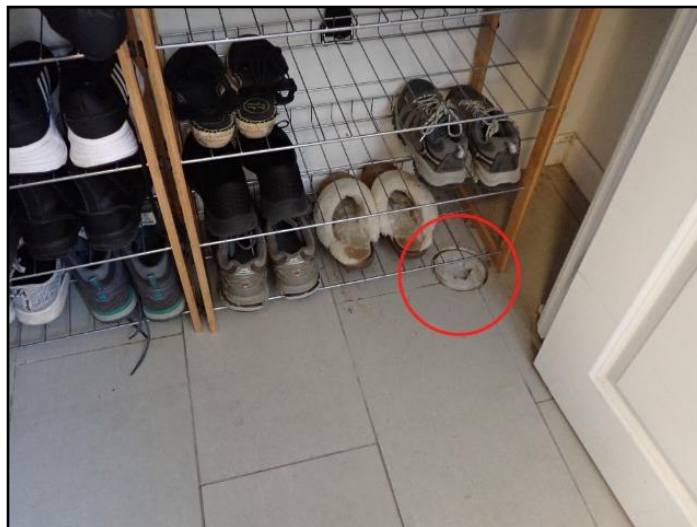
Plastic cleanouts often indicate drain work
