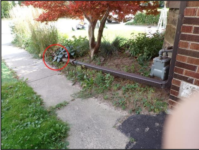
Maintain discharge well away from foundation
