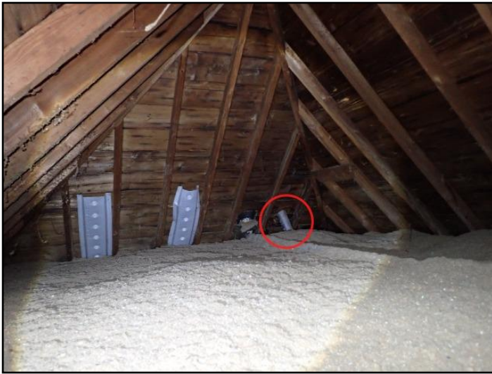
Ductwork not insulated in Attic
