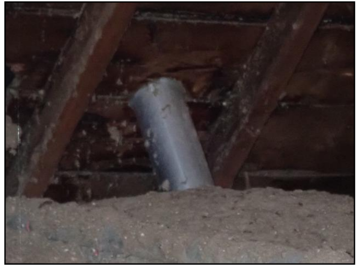
Ductwork not insulated in Attic
