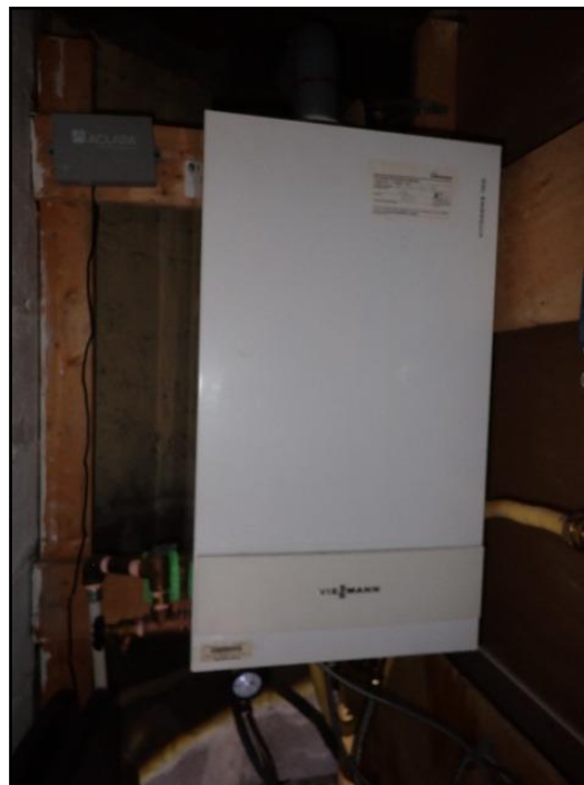
Boiler is approx. 16 years old
