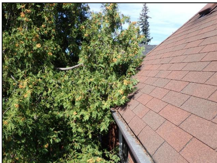
Tree branches touching roof
