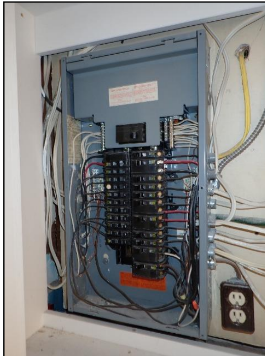
Panel and wiring are in good condition
