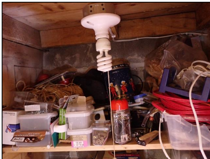
Exposed to mechanical damage (No cage or...
