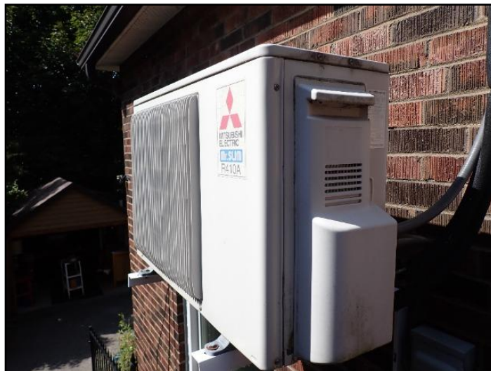
Heat pump is approx. 16 years old
