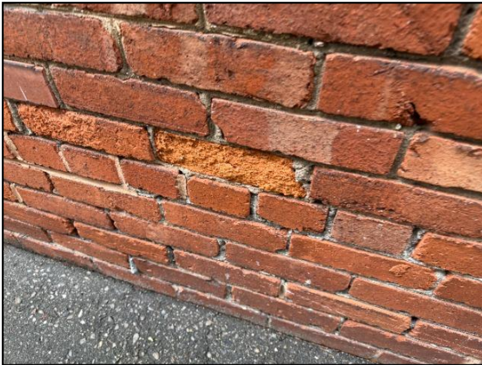
6. one example of spalling
