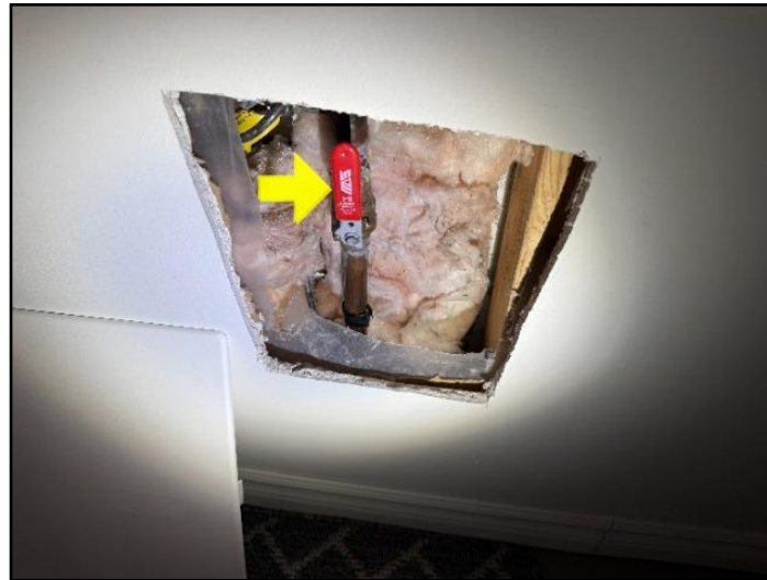
14. Main water shut off valve - Basement
