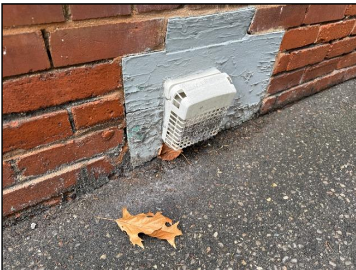
4. Vent near grade
