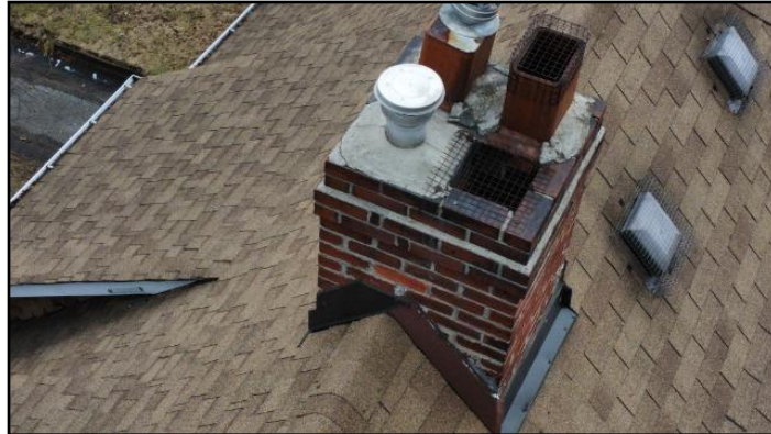
13. No drip edge on cap (crown)
