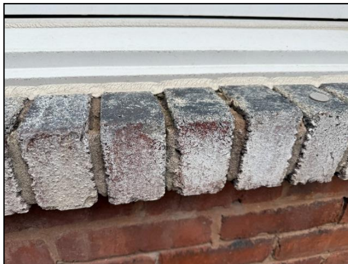
8. example of mortar deterioration at sill
