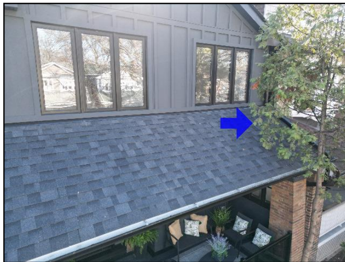
Tree branches touching roof
