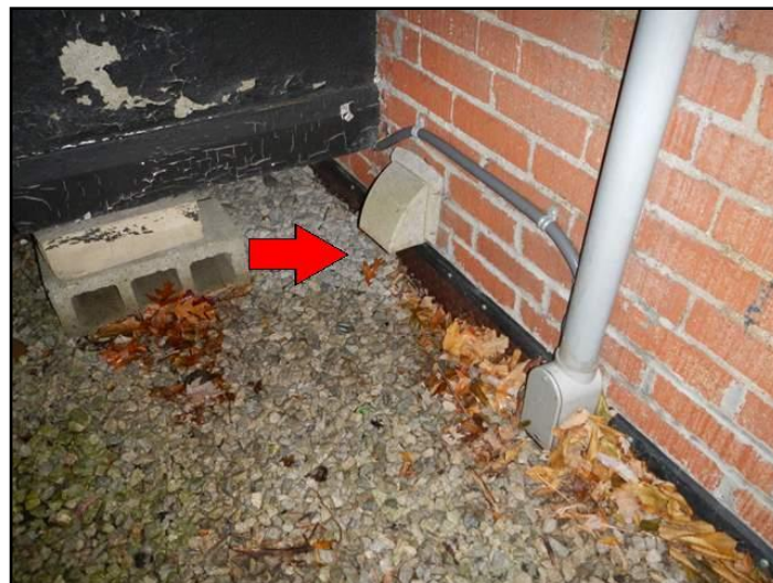
Too close to grade
