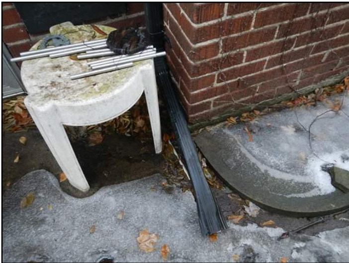
Discharge too close to building
