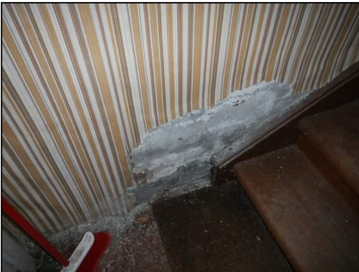
Damage: basement walkout
