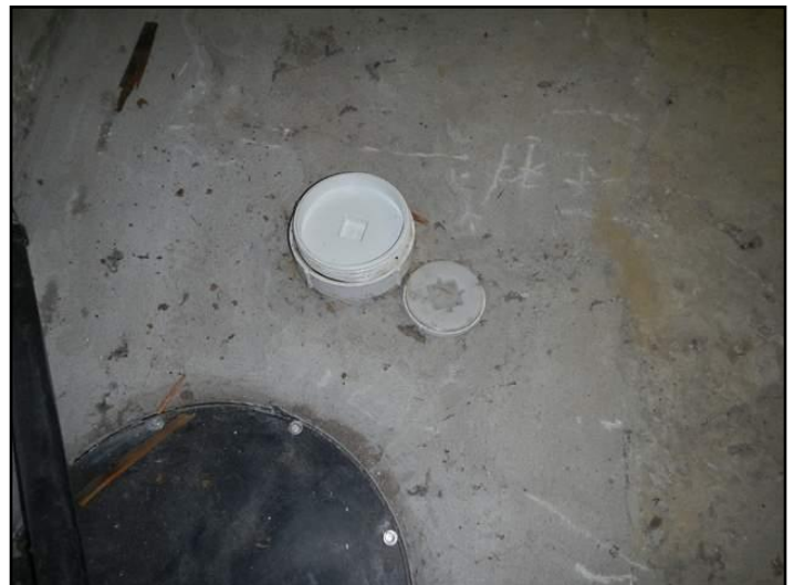
Plastic in the boiler room
