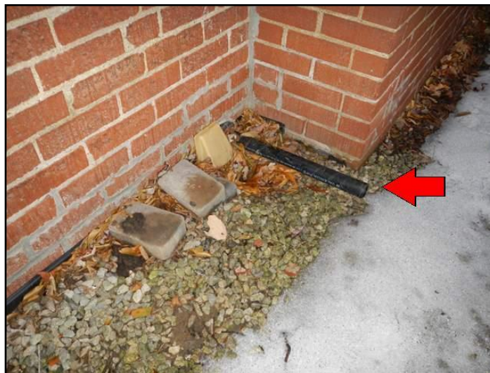
Discharges less than 6 feet from home
