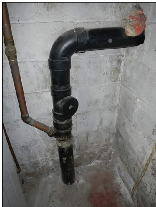
Plastic in the boiler room
