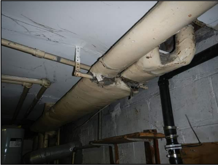
Insulation on boiler piping
