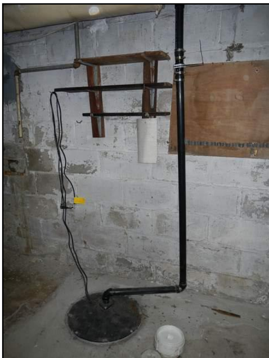
Sump pump in boiler room.
