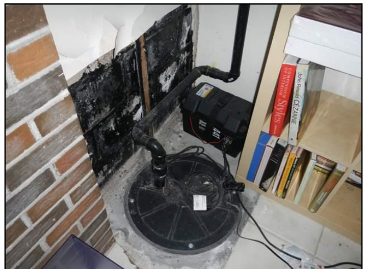
In Rear living room, with backup battery.
