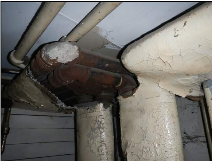
Insulation on boiler piping
