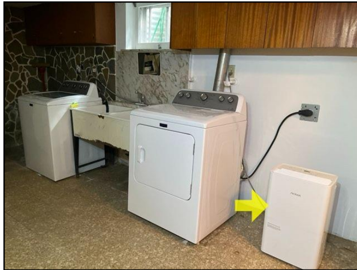
Dehumidifier in basement
