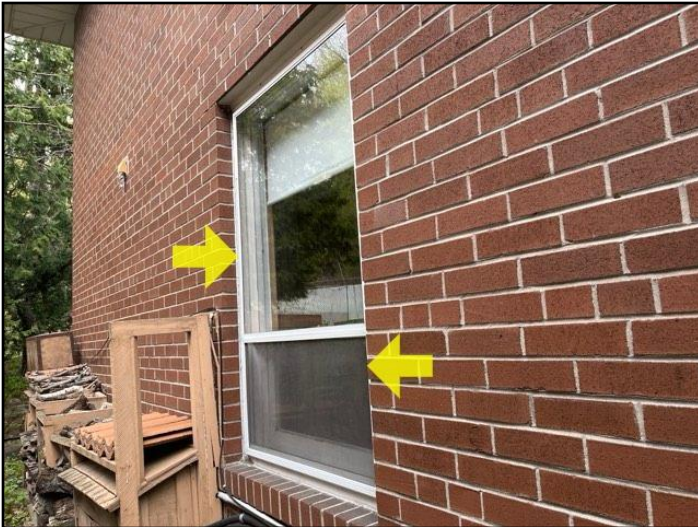
Ex., Left side: Caulking deteriorated
