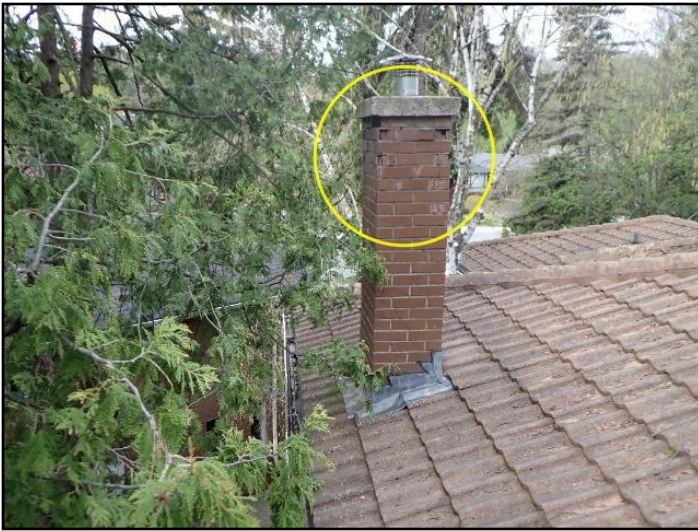
Example, Right side: Loose, Missing Masonry
