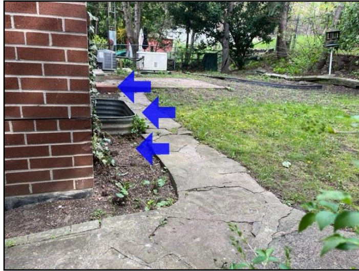
Improper slope or drainage
