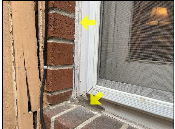
Detail: Caulking deteriorated
