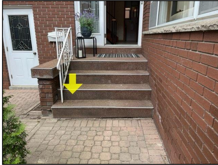
Steps or landings settling or heaving
