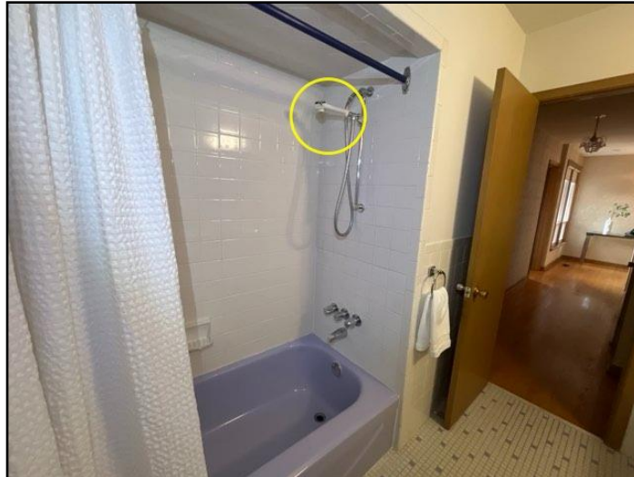
Leaky hand shower
