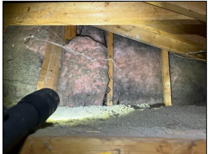
Fiberglass on Walls
