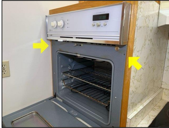
Not well secured
