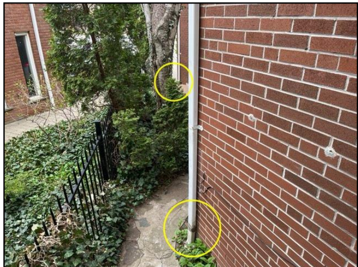
Toronto - Discharge below grade
