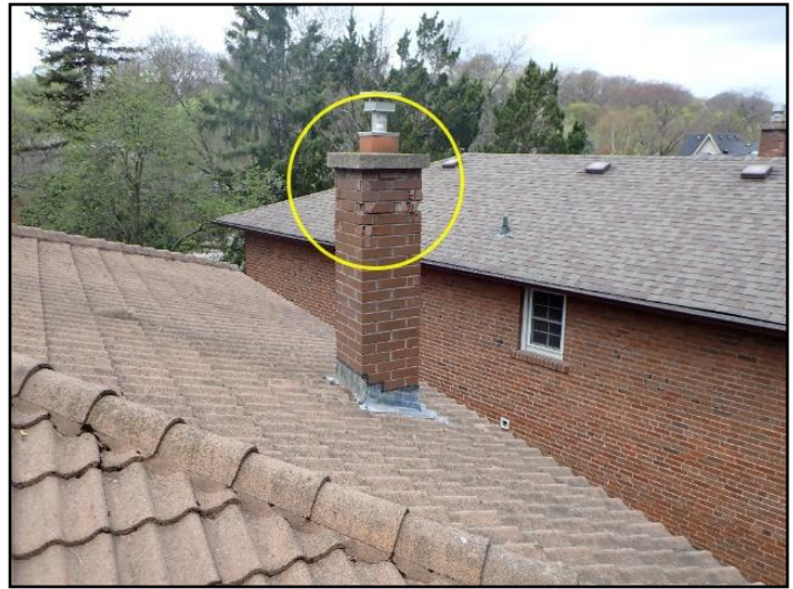
Example, Left side: Loose, Missing Masonry
