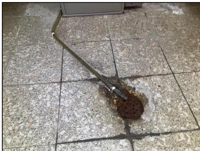
Grate missing, rusted or obstructed
