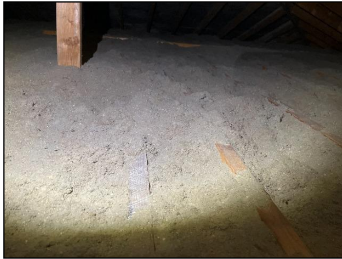
Amount less than current standards
