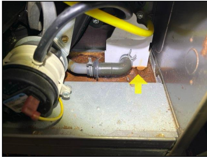
Condensate leak - active
