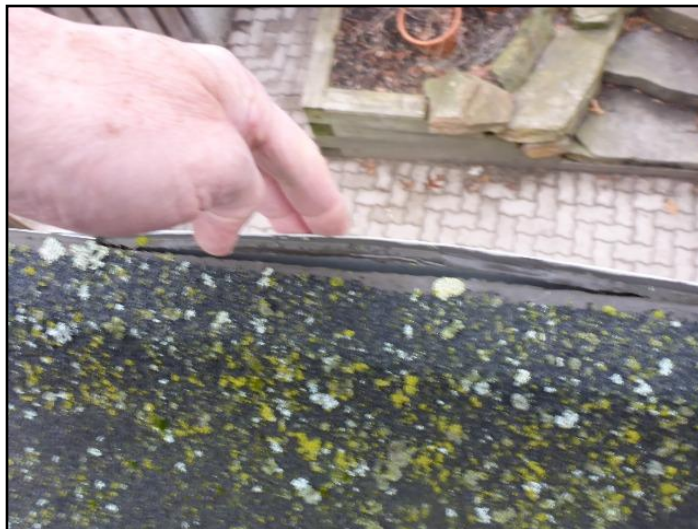
Edges, seams and/or flashings - loose, open
