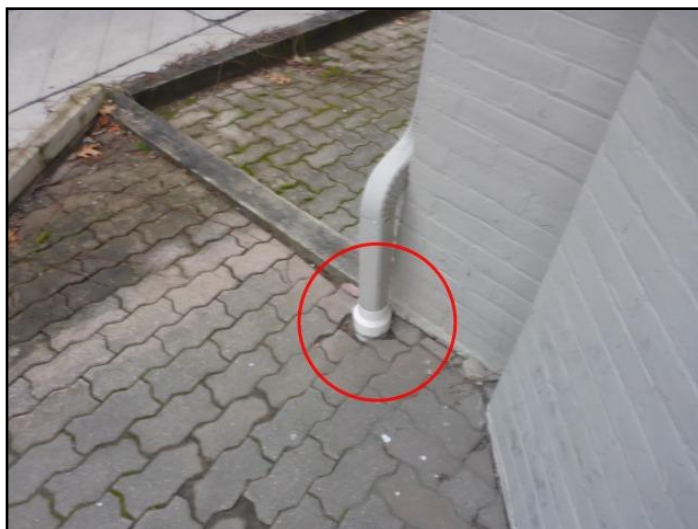
Discharges to front yard
