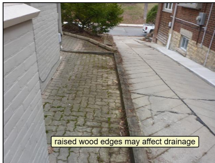
Improper slope or drainage
