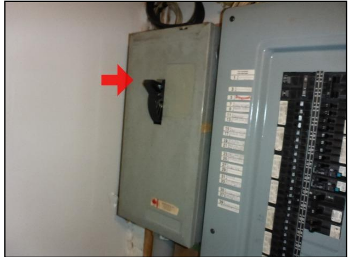
Main electrical disconnect indicated
