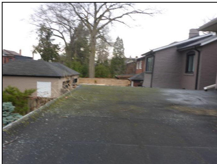
Moss on flat roof
