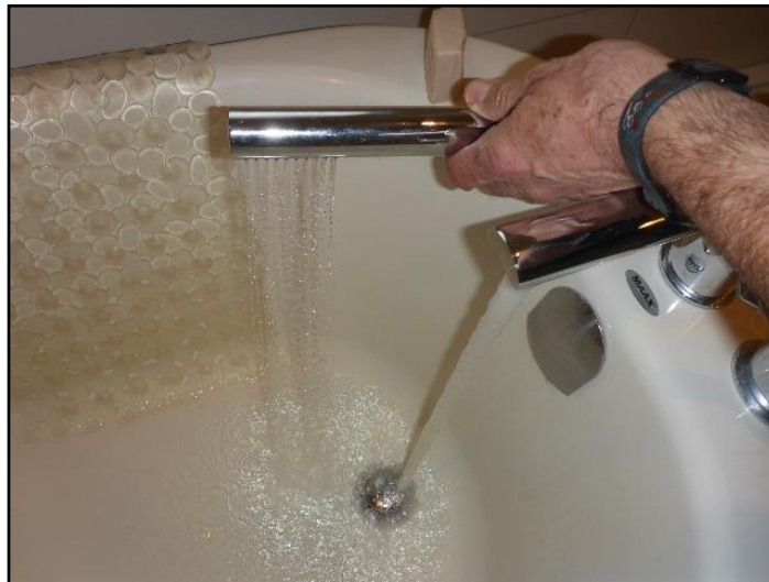
Shower diverter inoperative / ineffective
