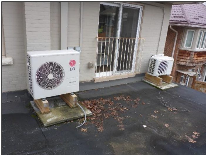
Ductless (Mini split) system- outdoor units
