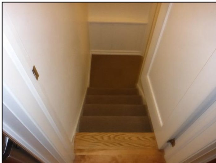
Incomplete or not continuous railing
