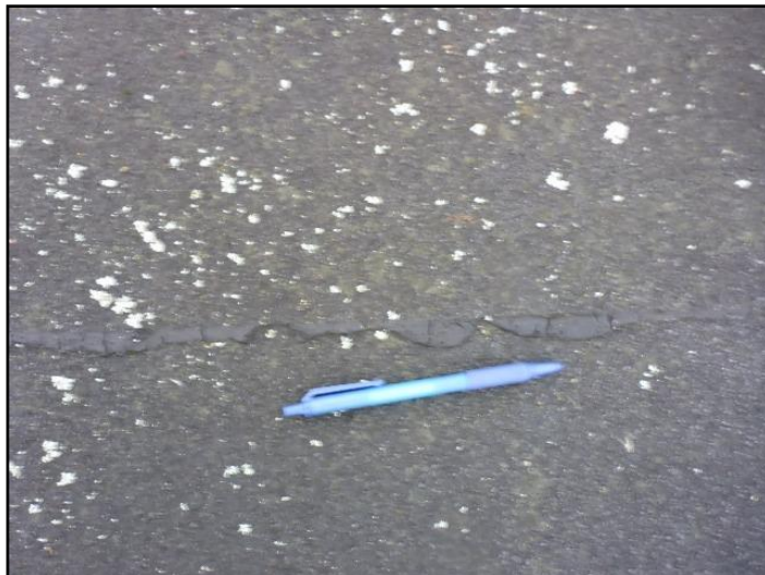
Cracks noted in tar seams
