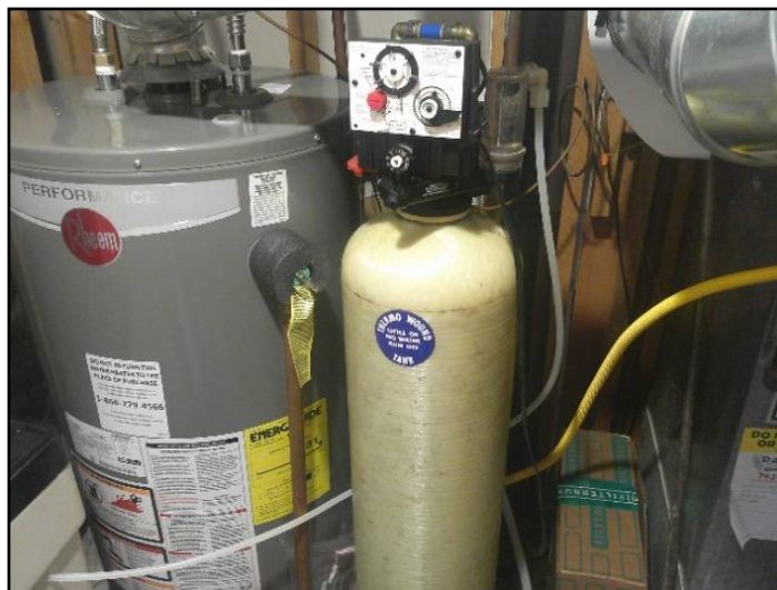
41. Water softener noted
