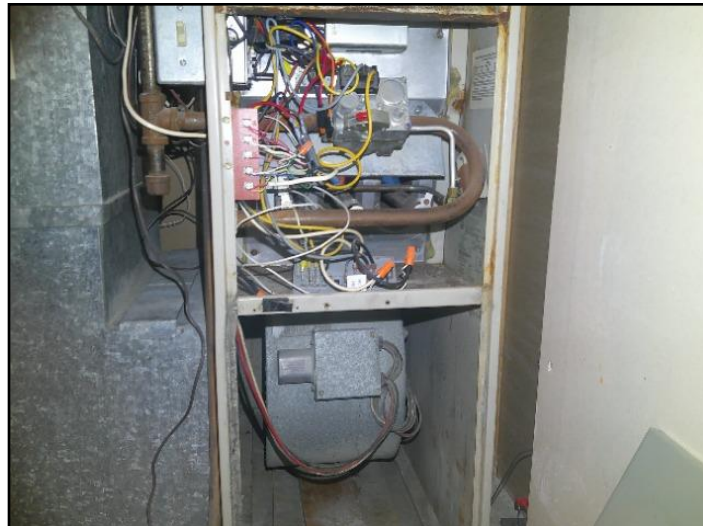
18. Furnace cabinet inspected
