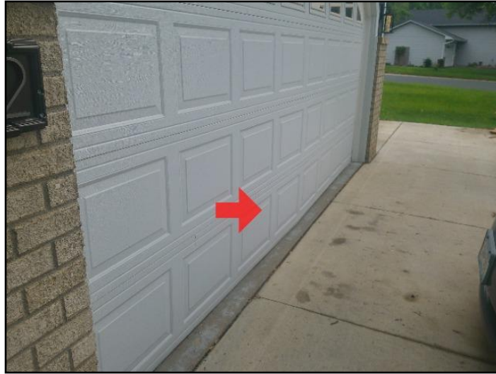
12. Dented / Bulging garage door
