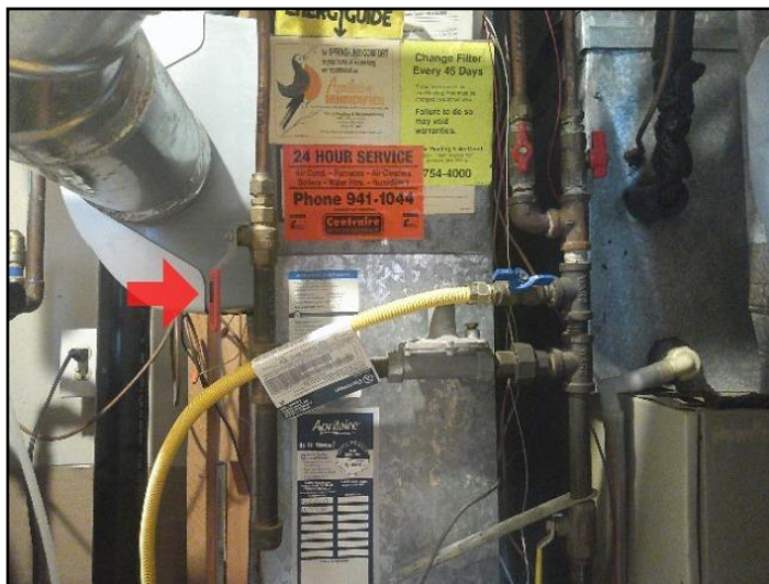
43. Main gas shutoff valve
