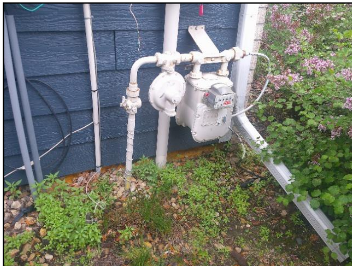
42. Exterior left side gas meter
