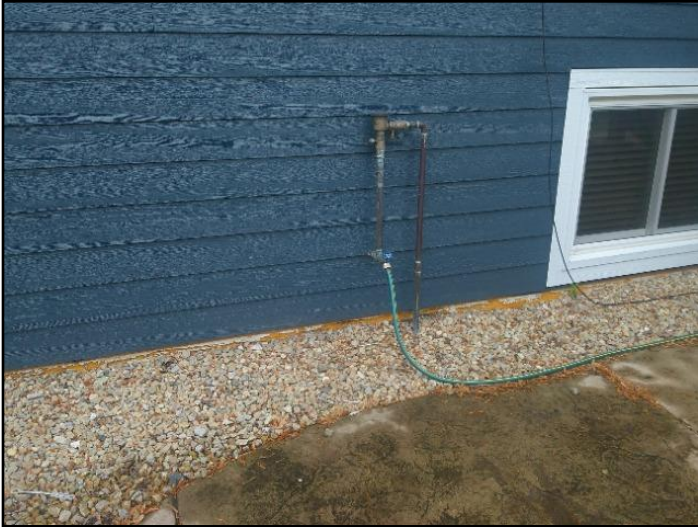
44. Landscape irrigation system
