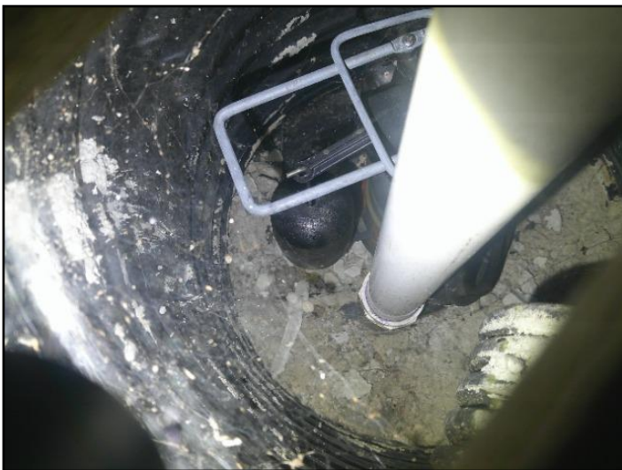
39. Sump pump basket is dry
