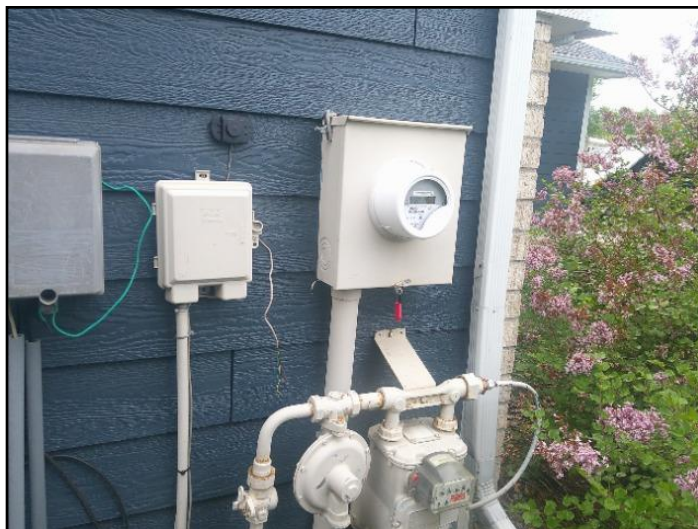
13. Underground aluminum service entrance
