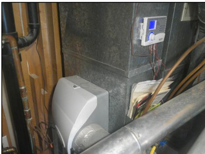
23. Duct mounted bypass humidifer
