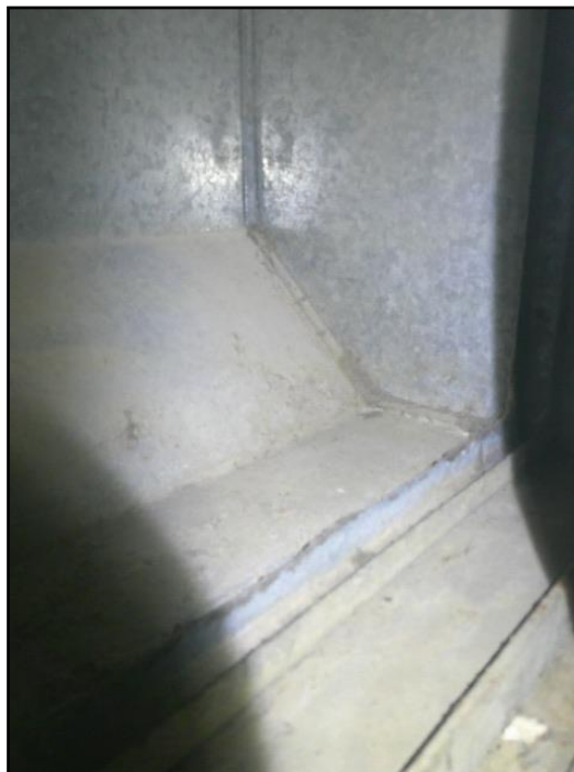
25. Ductwork due for cleaning
