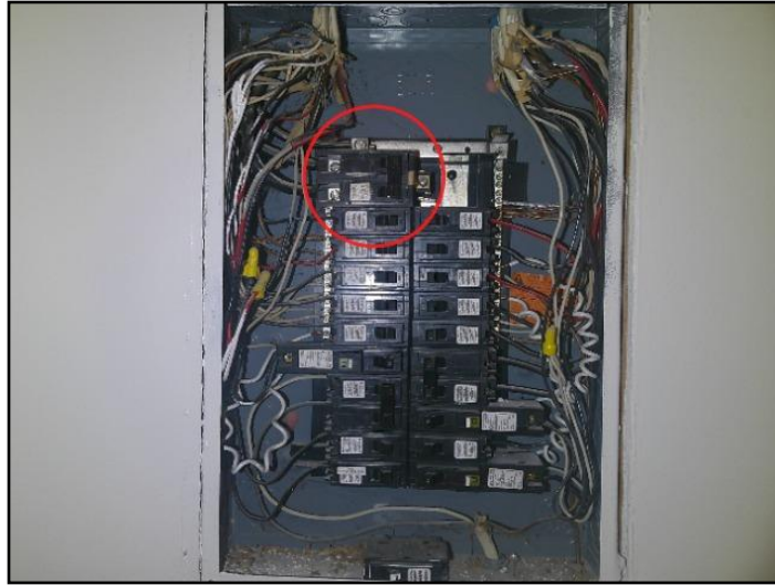
16. Main disconnect breaker
