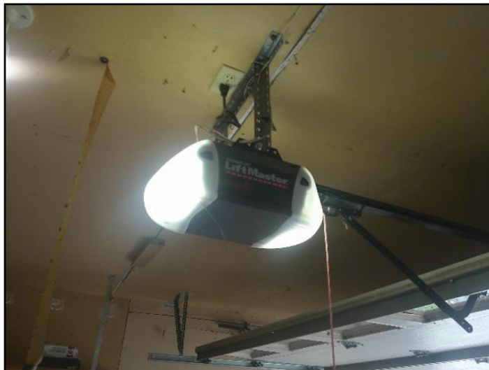
57. Chamberlain/LiftMaster door operator tested
