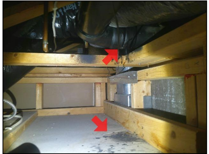
63. Previous leak from toilet drain
