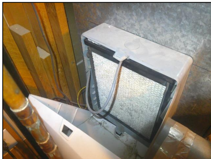
24. Duct mounted bypass humidifer
