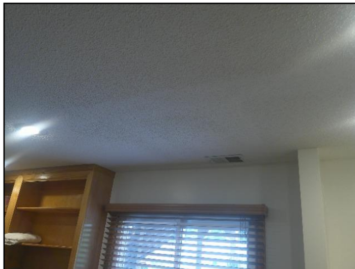
61. Patched ceiling below kitchen sink
