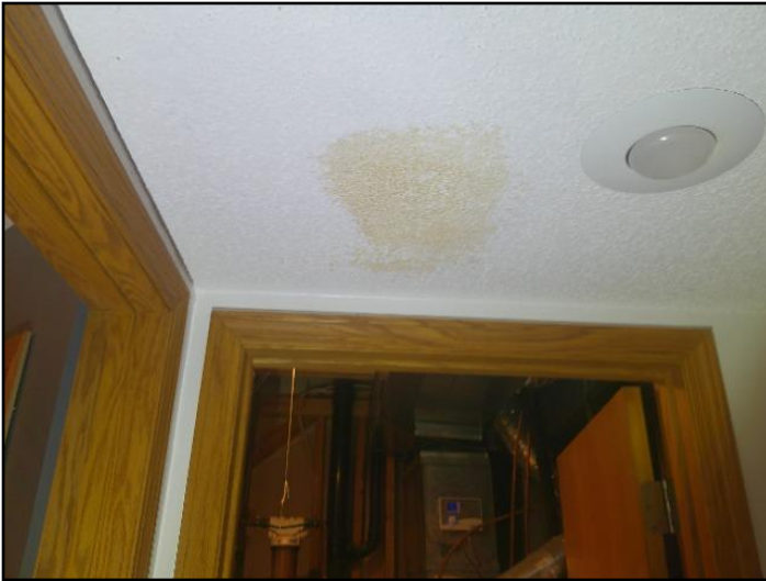
62. Water stains on ceiling
