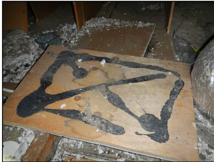
Not insulated and not weatherstripped
