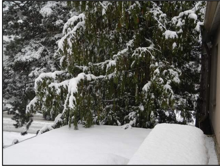
Tree branches touching roof
