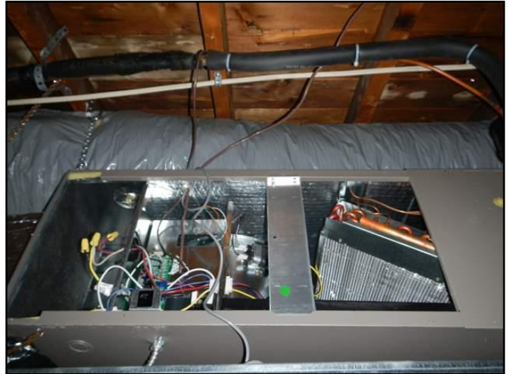
Air handler in the attic.
