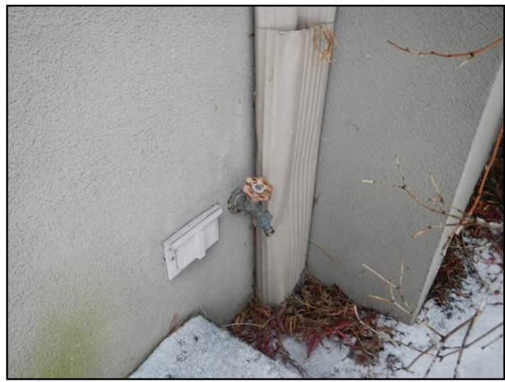
Toronto - Discharge below grade
