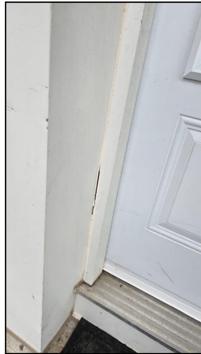
14. Caulking missing, deteriorated or loose
