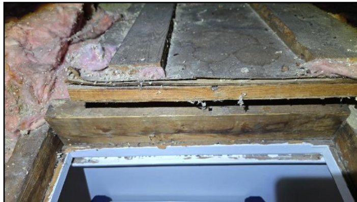
85. Not insulated and not weatherstripped
