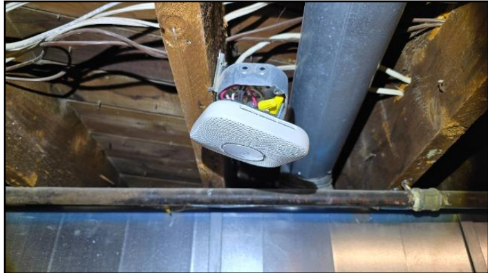
49. Recommend securing smoke detector
