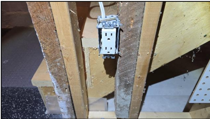
46. Damaged, loose or missing
