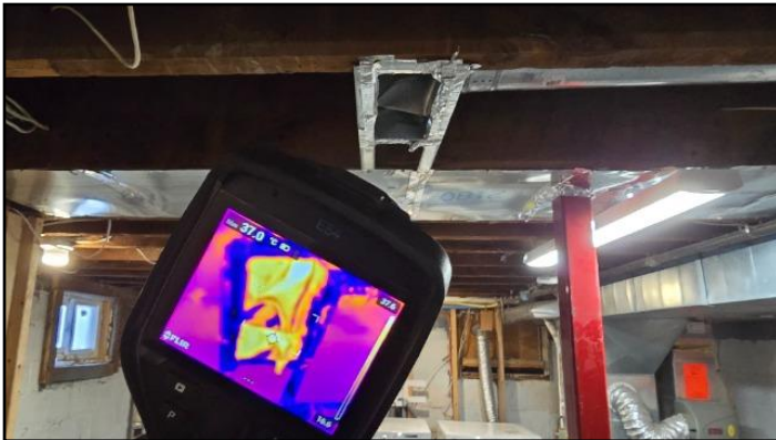
68. Ducts and registers
