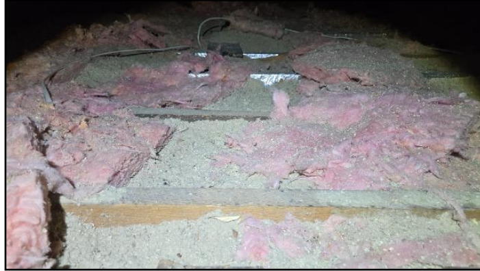
84. Amount less than current standards
