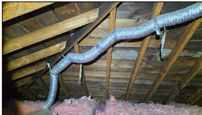
106. Not insulated in unconditioned space
