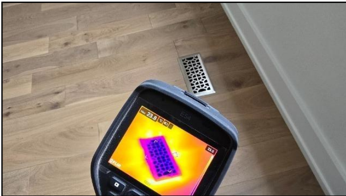
70. Ducts and registers
