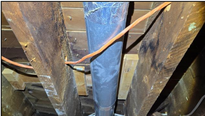
41. Too close to/touching ducts, pipe, chimneys...
