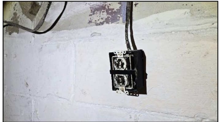
45. Damaged, loose or missing
