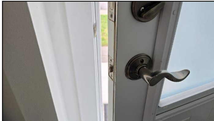
103. Latch not effective on exterior door
