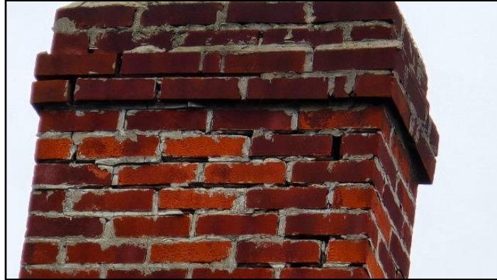
62. Loose, missing or deteriorated mortar
