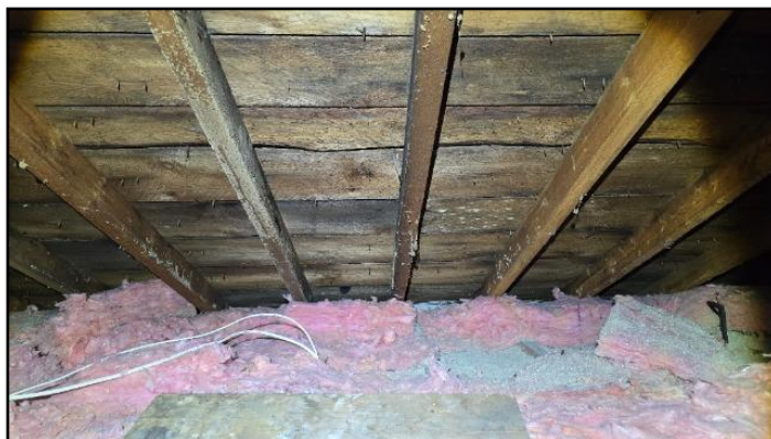
5. Vents - ineffective / missing
