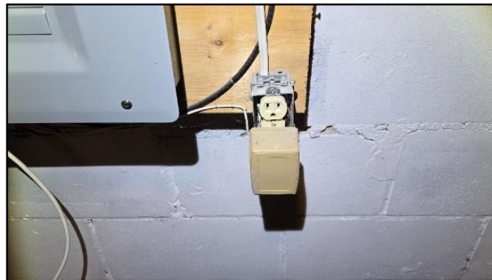
48. Damaged, loose or missing
