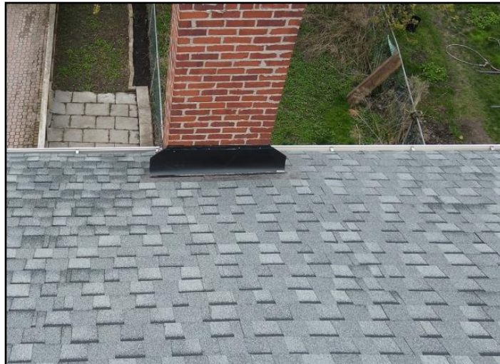
1. Cricket (Saddle) missing, loose, damaged
