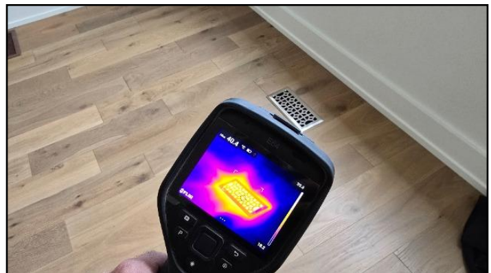
67. Ducts and registers
