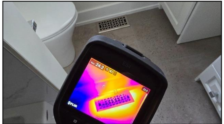
69. Ducts and registers
