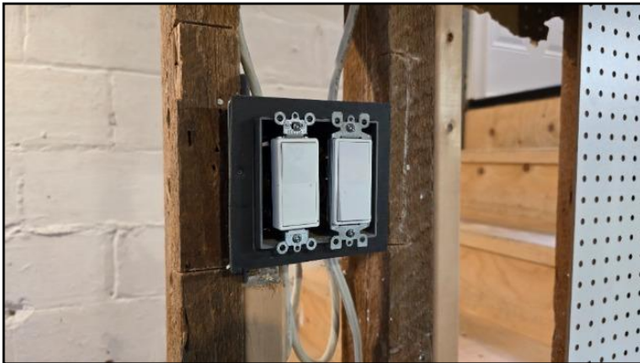
44. Damaged, loose or missing
