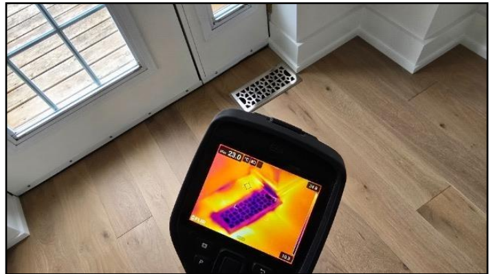
71. Ducts and registers
