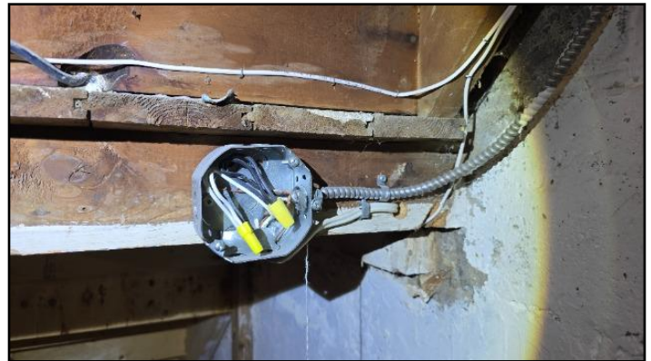
47. Damaged, loose or missing
